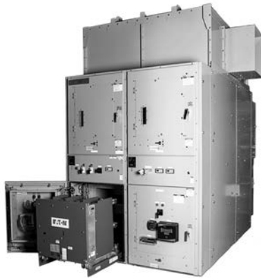
Arc-Resistant Switchgear with Plenum Installed
