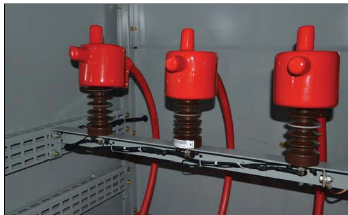
Figure 5.5-5. OVS Sensors Mounted in Cable Compartment
