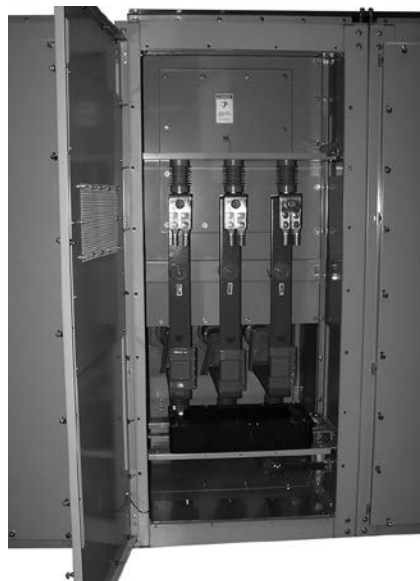
Rear View—Typical 27 kV Breaker Cable Termination
