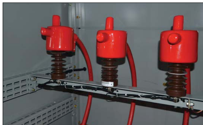
Figure 5.3-9. OVS Sensors Mounted in Cable Compartment
