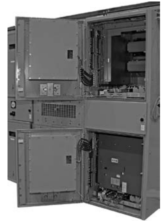
5/15 kV Breaker Over Breaker
