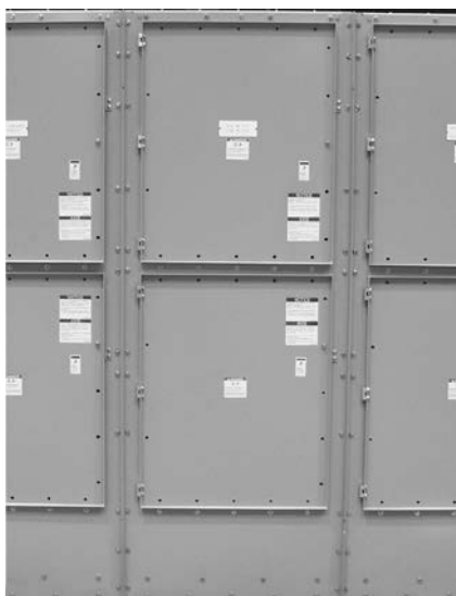
Rear View 5/15 kV VCP-W Arc-Resistant Switchgear
